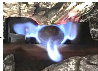
Inspect Pilot Flame
