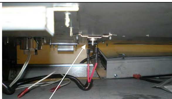
Thermodisc is located in track under firebox.
