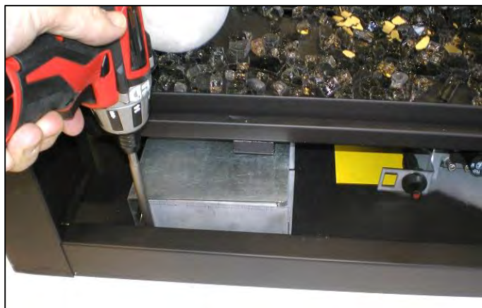
Power Vent Control Module Mounted inside fireplace.
